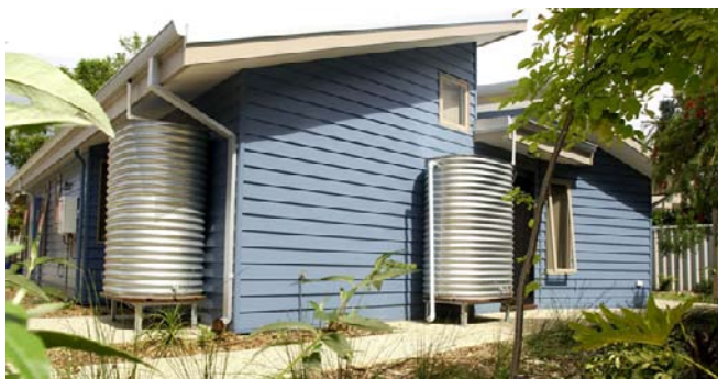
Eastern garden grey water irrigation and eaves tanks
